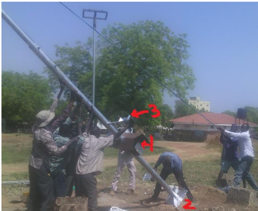
Figure 1 Attaching the 10m Node to the base, already fixed by concrete (1, indicates the cage for the gateway, 2 indicates the base of the stand, 3 shows an interface for attaching the 2m node)
